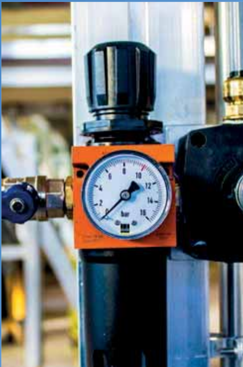
Druckluftanschlüsse Compressed air connections
